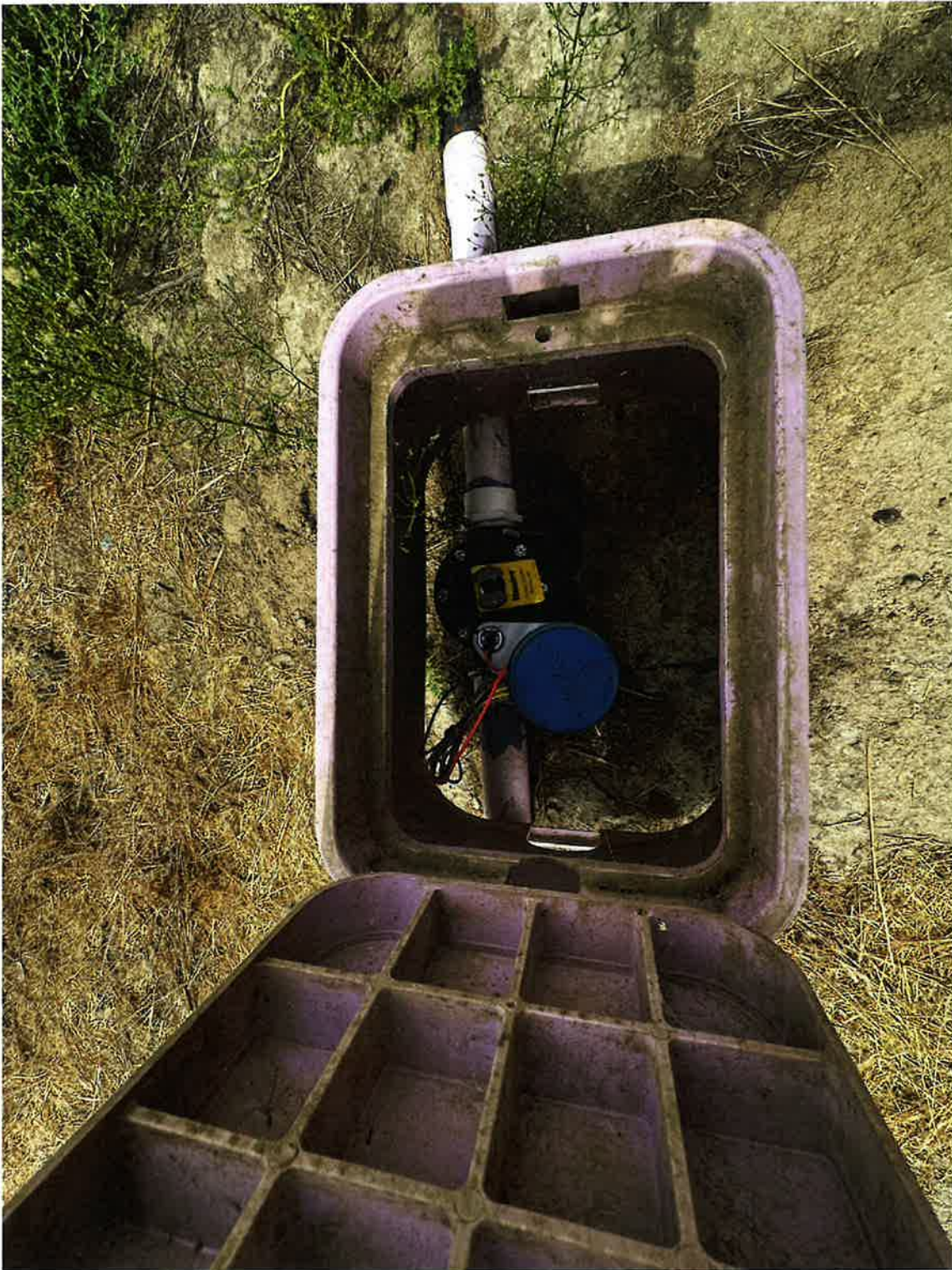
New automated water valve at the habitat mitigation area.
