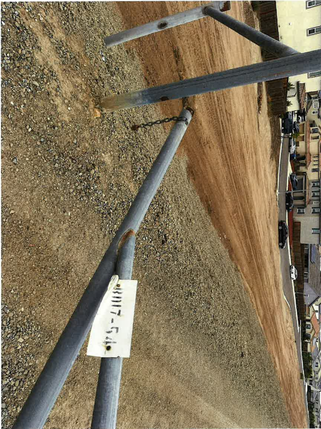
Sta 945+00 - Damaged gate chain, to be repaired.
